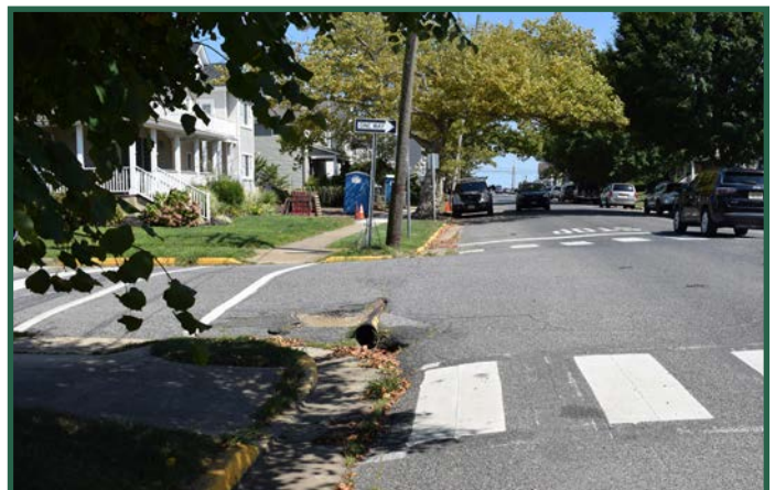
Figure 47. Exposed drain pipe at B Street.
