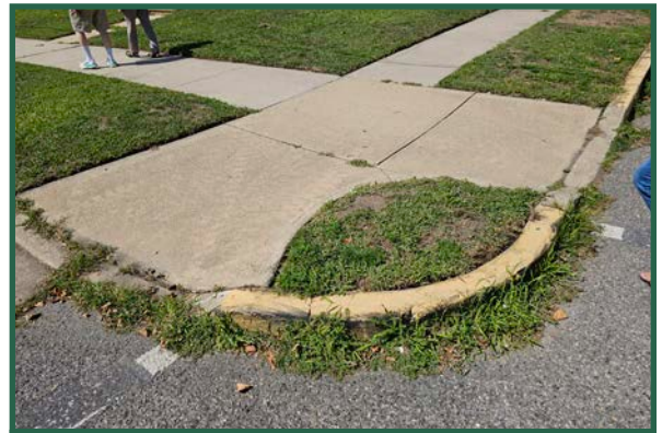
Figure 44. Non-compliant curb ramps.
