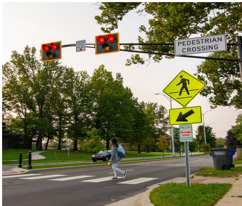
Figure 3. A PHB installed at Washington Street, Kokomo, IN (IUK, 2020)
