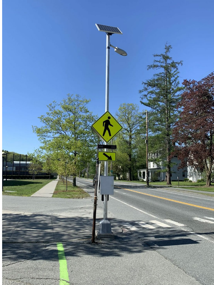
Figure 14. An overhead lighting (Carmanah, 2022)
