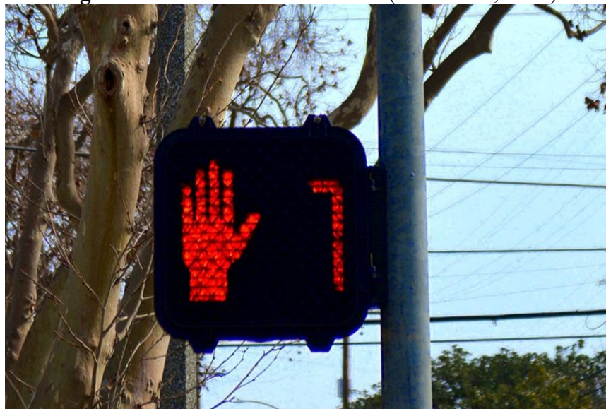
Figure 6. A PCS installed in Long Beach, CA (Longbeach, 2022)
