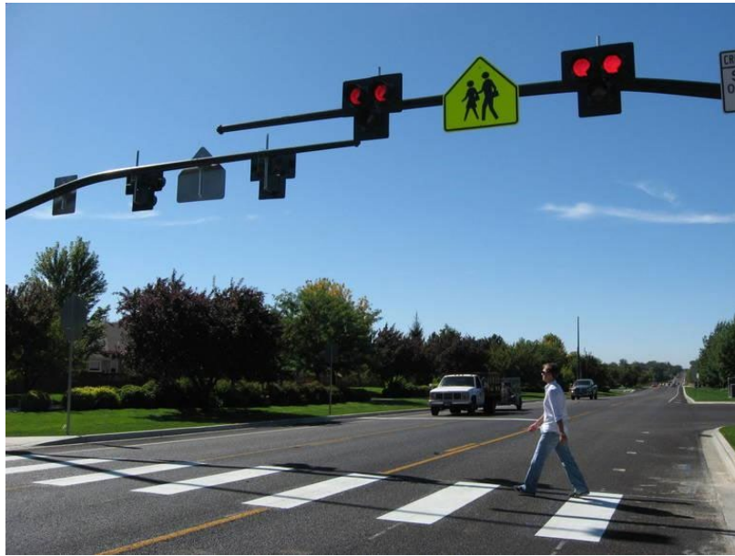
Figure 2. A PHB installed at Maple Avenue, Plainfield, NJ (TAPINTO, 2019)
