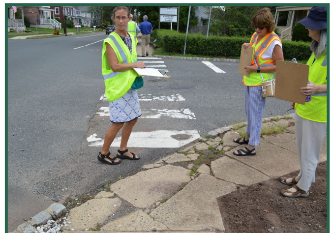
Figure 44. Broken curb ramp.
