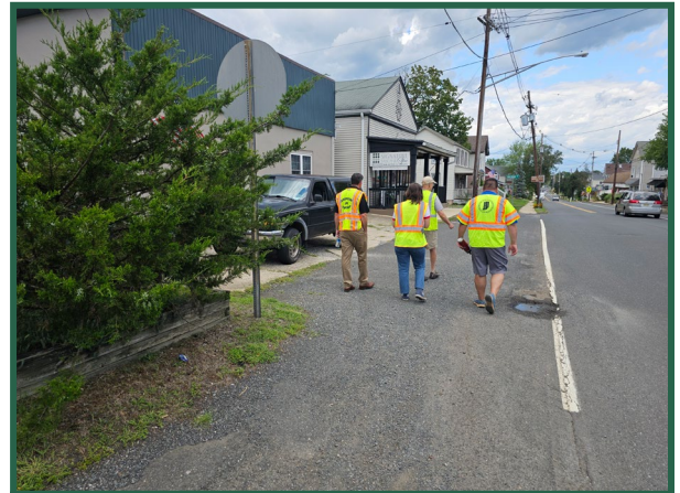
Figure 16. Missing sidewalk in front of 153 Main Street.
