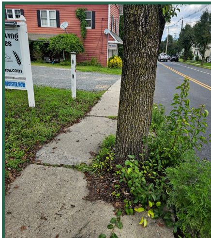
Figure 19. Sidewalk broken by tree roots.
