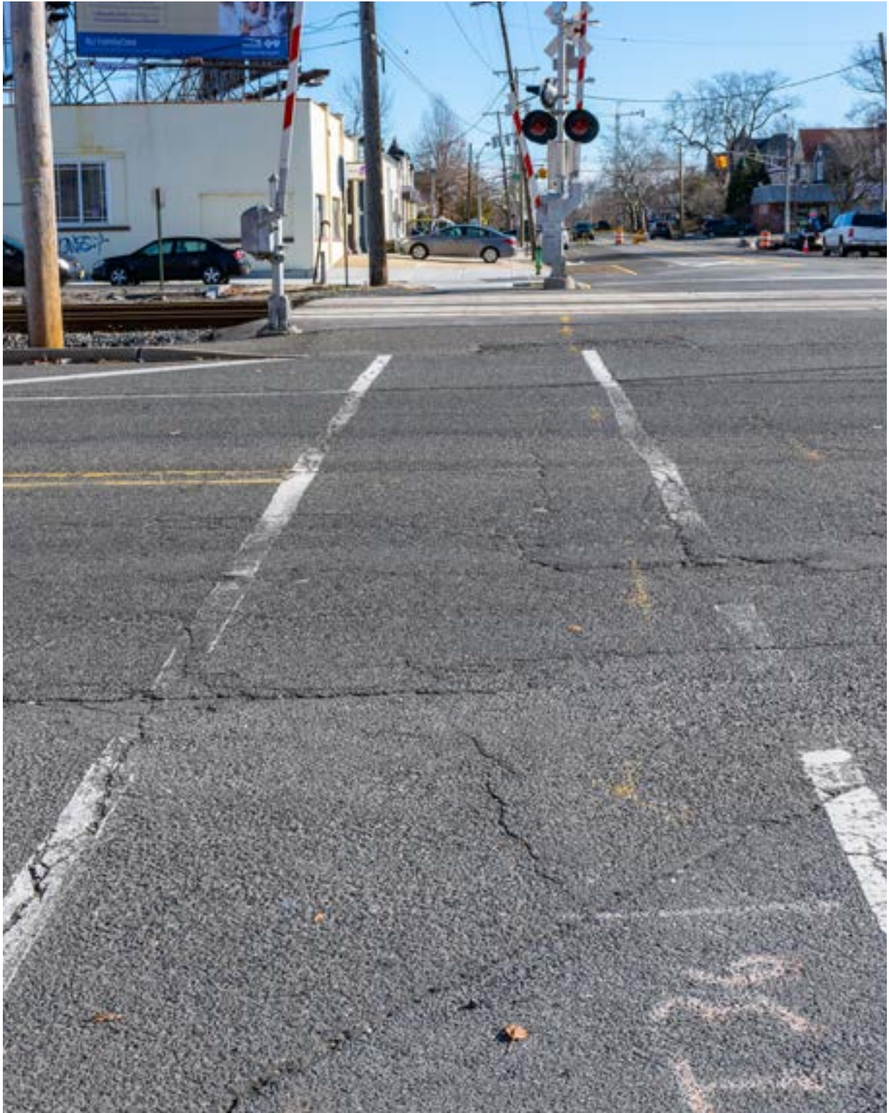
Most Memorial Dr crossings lack highly visible crosswalks and ADA compliant curb ramps. Additionally, crossings are long and unpredictable due to the offset stop bars and railroad tracks
