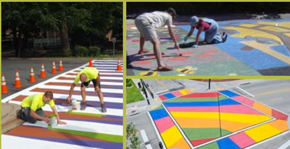
(clockwise from top right) Residents installing a painted intersection in Boulder, CO ( www.bouldercolorado.gov ); painted intersection in Ft. Lauderdale, FL ( www.fortlauderdale.gov ); colorful crosswalk in Silver Springs, MD ( www.montgomeryplanning.org )
