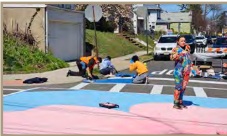
Figure 28. Additional views of the installation.
