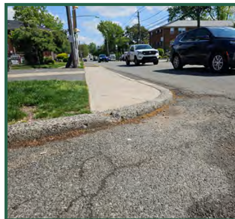
Figure 66. Missing curb ramp.
