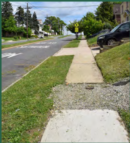
Figure 75. Broken sidewalk on Greylock.
