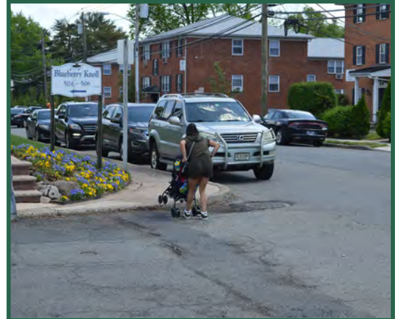
Figure 77. Missing curb ramps on Joralemon Street.
