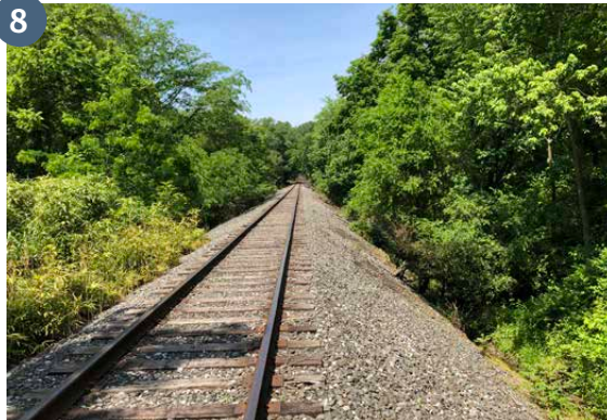
Significant ballasting west of N. Coles Avenue in Maple Shade.
