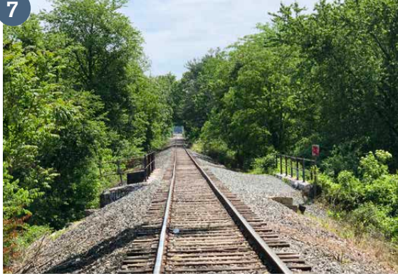
The study area rail corridor crosses South Branch Pennsauken Creek (border of Pennsauken and Maple Shade) over a large double arch culvert structure (view east).
