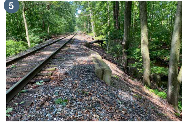
5 Large culvert at South Branch Pennsauken Creek Tributary in Pennsauken (view west).
