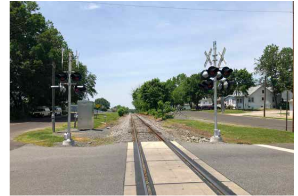
Recent upgrades at Stiles Avenue include new crossbucks with flashing lights along with a new control box.
