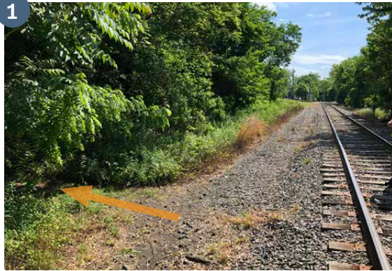
1 Existing informal path between P.Y.A.A. Park/Brey Memorial Field and the study area rail corridor at the western end of the study area (view east).
