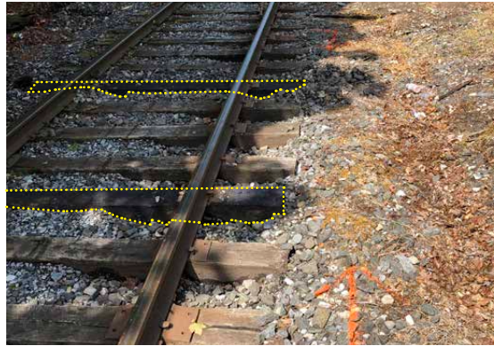
Orange markings surround an area where two railroad ties (indicated in yellow) were recently replaced.
