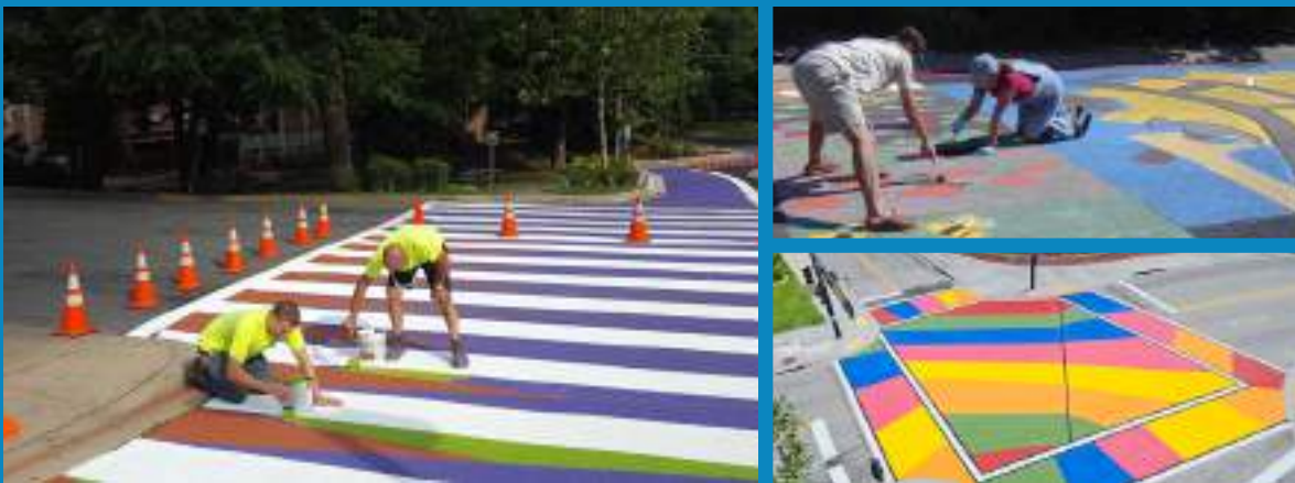
(clockwise from top right) Residents installing a painted intersection in Boulder, CO ( www.bouldercolorado.gov ); painted intersection in Ft. Lauderdale, FL ( www.fortlauderdale.gov ); colorful crosswalk in Silver Springs, MD ( www.montgomeryplanning.org )
