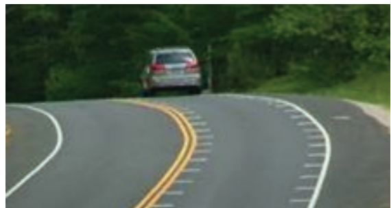
Example of paint speed reduction markings
