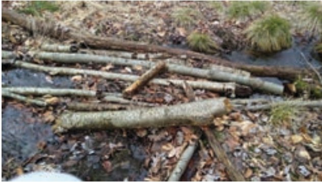
Log Bridge / area in need of repair
