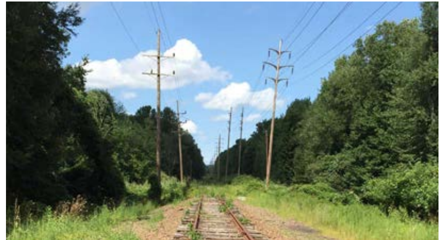
Example of overhead distribution lines on the east and west sides of the study area right-of-way (view north from Blanch Avenue in Closter).
