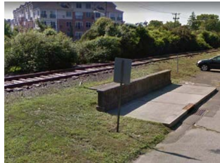
Headwall of culvert at Tenakill Brook Tributary in Tenafly (identified in Map 2.4 as item C-3).
