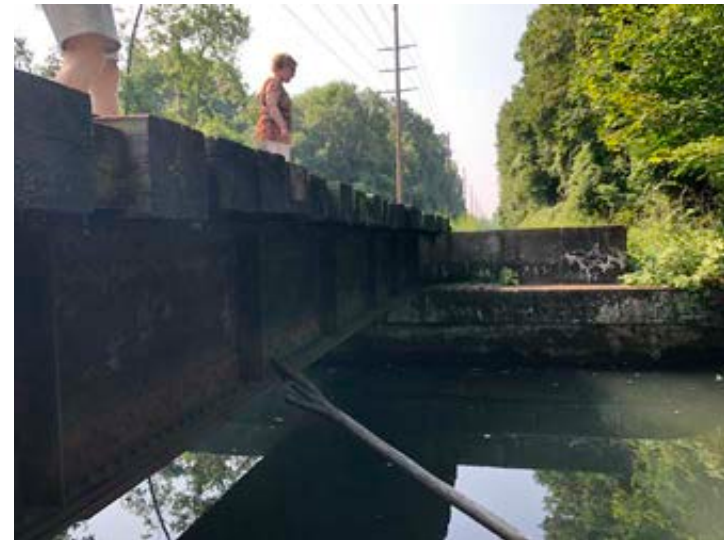
Steel girder bridge with concrete abutment spanning the Tenakill Brook in Demarest (identified in Map 2.4 as item B-2).
