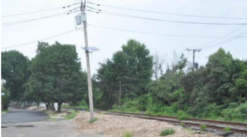
Example of distribution lines within the study area in Tenafly (near Tenakill Swim Club).
