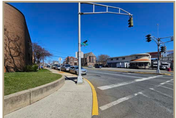
Figure 13. Old traffic signal, non ADA-compliant ramp, and narrow sidewalk outside City Hall.
