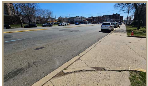
Figure 14. Narrow sidewalk with degraded concrete at City Hall driveway.
