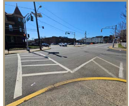
Figure 18. Looking southeast, the curb ramps are not ADA-compliant.
