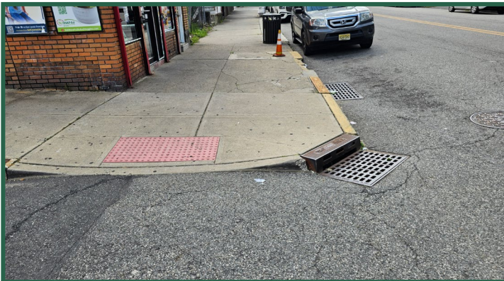
Figure 25. Complaint curb ramp.
