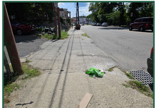
Figure 40. Driveway with uneven pavement.
