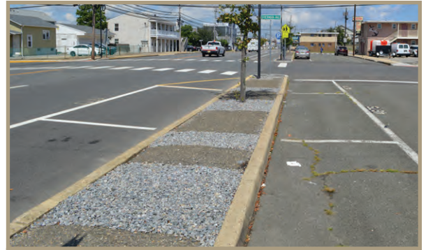
Figure 23. Empty tree wells and dying trees.
