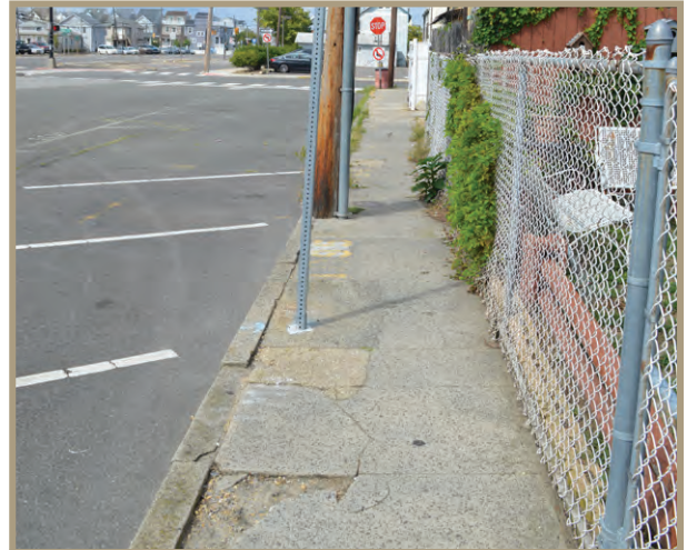
Figure 11. Narrow and cracked sidewalk with obstructions.
