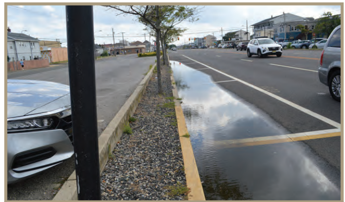
Figure 18. Poor drainage near intersection.
